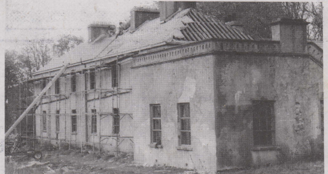
This magnificent old building could soon be alive again. Restoration work is in progress on the old Gweedore Hotel - an Chúirt.
