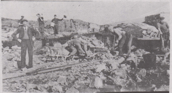
Work in progress on the laying-out of the Technical School, Lech an Iúir gardens in 1937.
